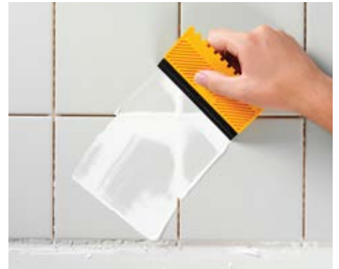
QUICSEAL 620 Durable Colour Grout fortified with QUICSEAL 609 latex – used to fill up the pointing gaps for all the tiling and marble works
