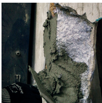
7 Use a trowel to apply the mixed QUICSEAL 515 to the prepared substrate
