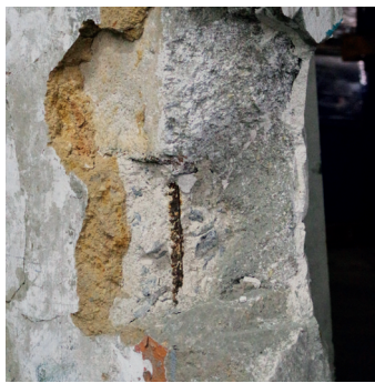
1 Corroded reinforcement observed behind spalling concrete
