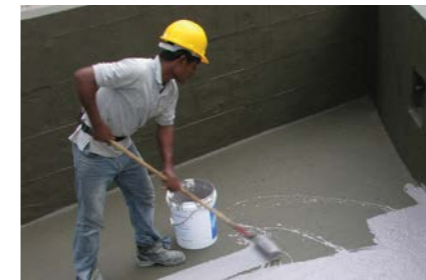
QUICSEAL 104 flexible cementitious system can be easily applied over large surface with airless spray, rollers or brush.
