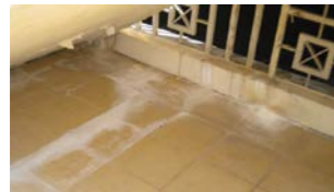
Efflorescence under staircase.
