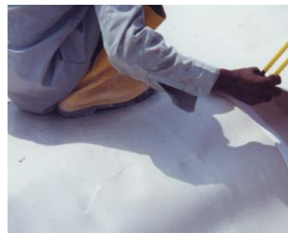
QUICSEAL 106 & 202 damp proof membrane and jointing tape used on foundation for moisture protection.
